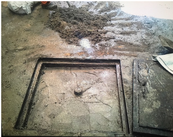
Relleno Cavity pz16-0024
